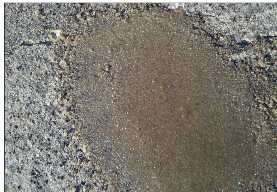
Pit patched with epoxy and sand
